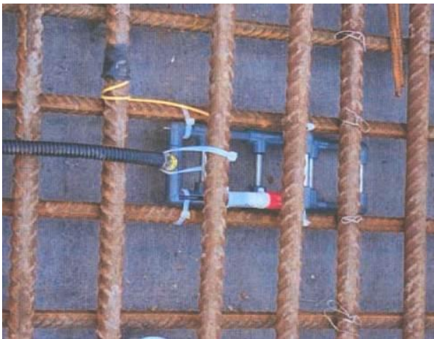
Fig.8: Corrosion sensors for monitoring of corrosion.
